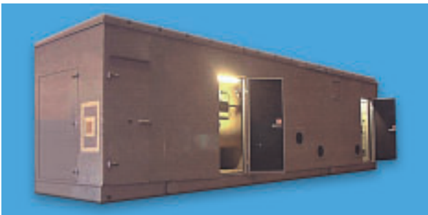
Chiller installed in AAF enclosure
